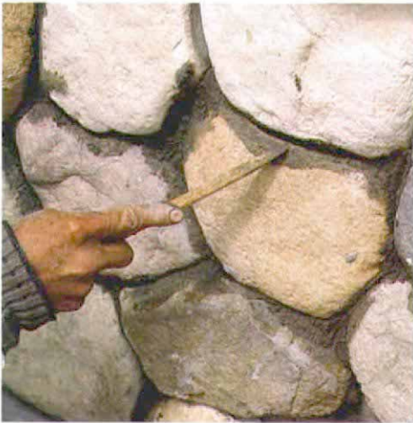
Cleanup begins with a small stick. When mortar has just begun to set up, a small softwood stick is used to remove excess. The pointed end rakes the joints between stones to the right shape and depth.
